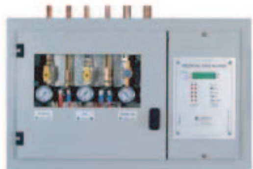
ASVU Box of 3 gases O_2 , Air, Vac with alarm
