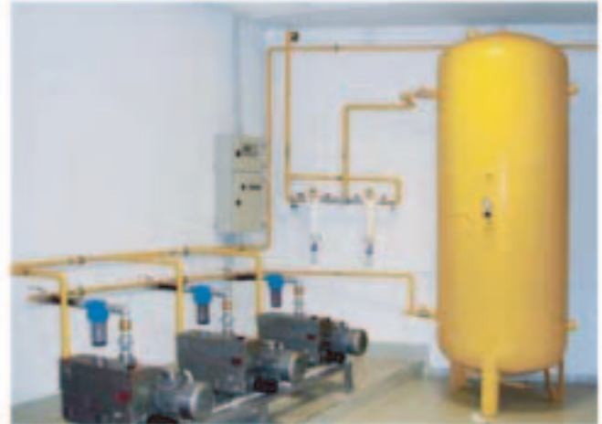
Medical Vacuum central station Horizontal
