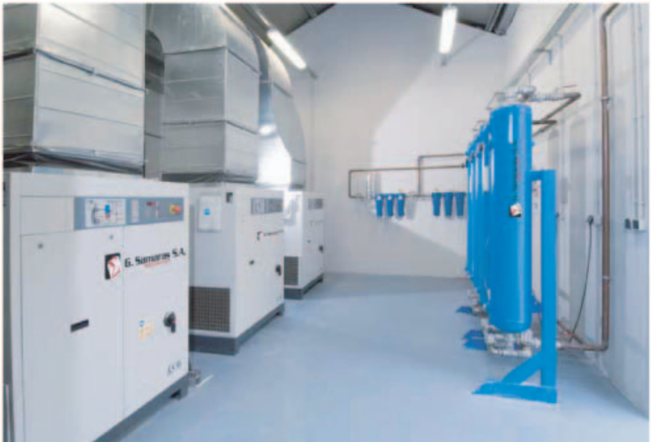
Medical Air central station
