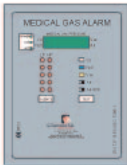
5gases alarm panel
